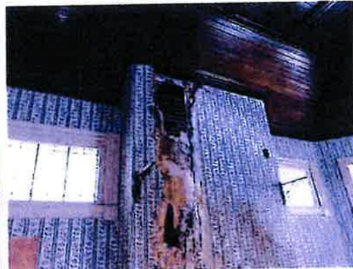
Water damage in living room
